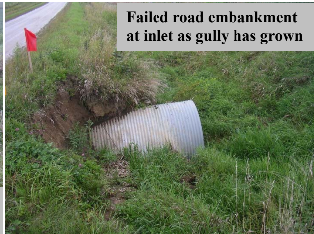
Looking at gully headcut from road
