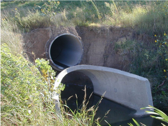
Photo 1. Storm Drain Conduits Need Restrained Joints
