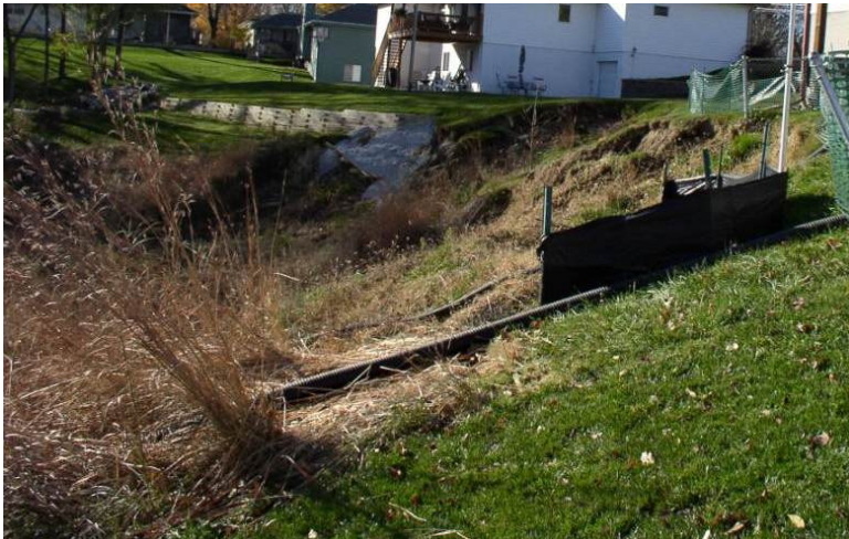
Photo 3. Uncontrolled Overland Flow
