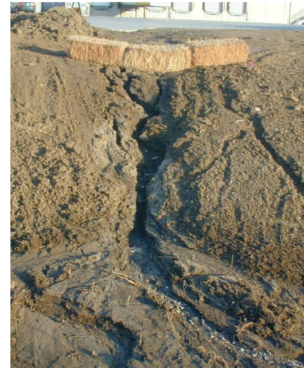
Photo 4. Uncontrolled Overland Flow
