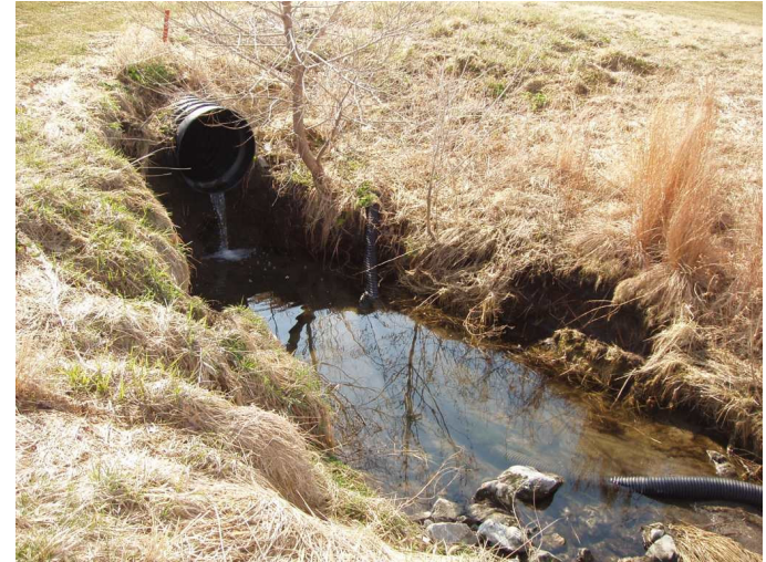
Photo 2. Outlets require erosion protection
