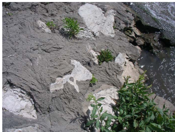
Photo of grouted limestone riprap on a weir. Despite being built less than thirteen years ago, the white limestone riprap is flaking and crumbling apart. Even though the riprap was covered with concrete grout (the gray coating), the grout cannot prevent the breakdown of the riprap. Eventually the rock will completely weather away, leaving a ring of grout which will then collapse because it has nothing left to support it. As you look at the photos below, note how the rock and grout, if present, weathers and disappears at the water line, whereas riprap or grouted riprap higher up the streambanks remains in good condition.
